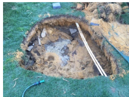
Not removing or decommissioning a septic tank
